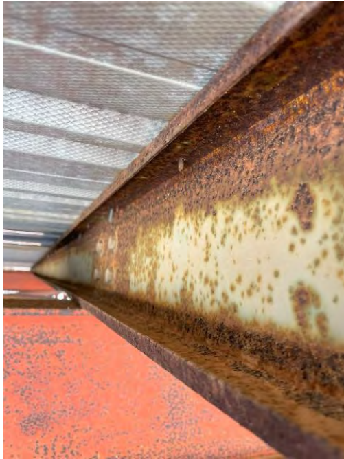
PICTURE 19 – TYPICAL PURLIN CORROSION EXAMPLE
