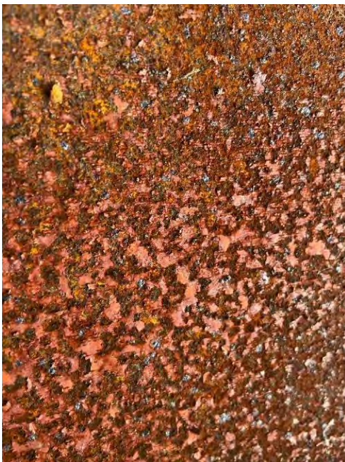
PICTURE 11 - EXAMPLE OF EXTENT OF CORROSION TO STEEL BEAM (SEVERE)
