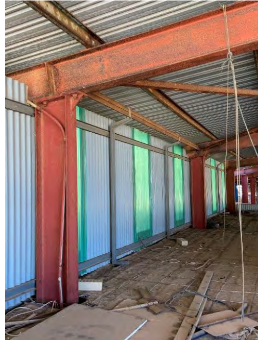
PICTURE 32 – COLLAPSED CEILING
