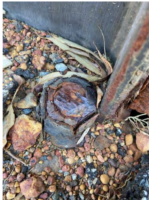
PICTURE 2 – CONDITION OF NUT AND THREAD – CORROSION MATERIAL IN PLACE
