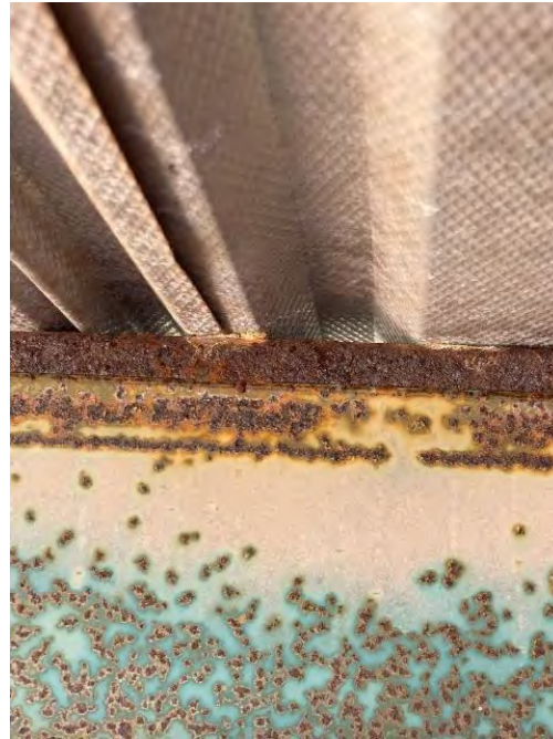
PICTURE 20 – TYPICAL PURLIN CORROSION EXAMPLE
