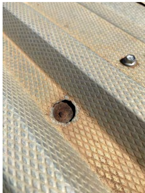
PICTURE 22 – GALVANIC CORROSION AT SCREW LOCATION.
