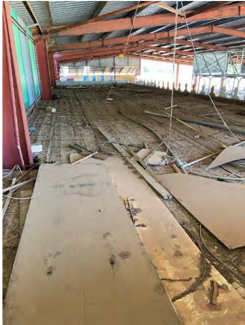
PICTURE 31 – COLLAPSED CEILING
