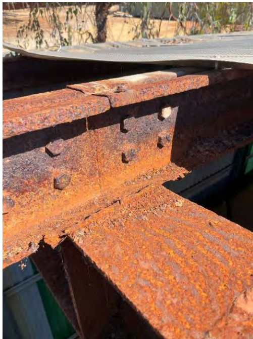
PICTURE 13 – SEVERE CORROSION TO PURLIN
