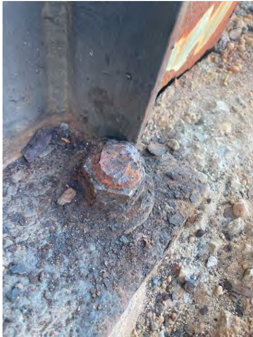
PICTURE 3 – CONDITION OF NUT WITH CORRODED MATERIAL REMOVED
